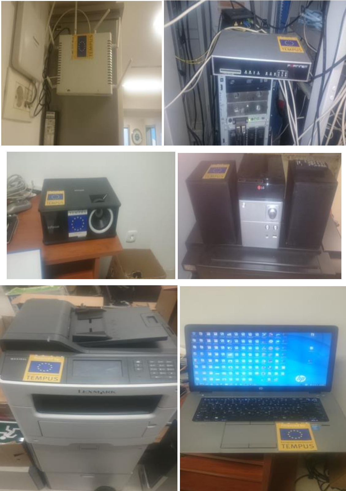
Picture 1. Equipment installed at Mediterranean University
